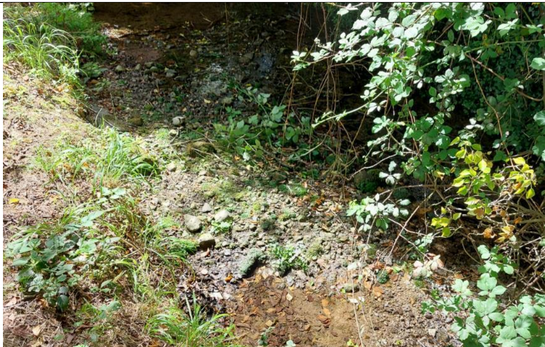
Erosion of the right bank of the Little Borris Stream.
