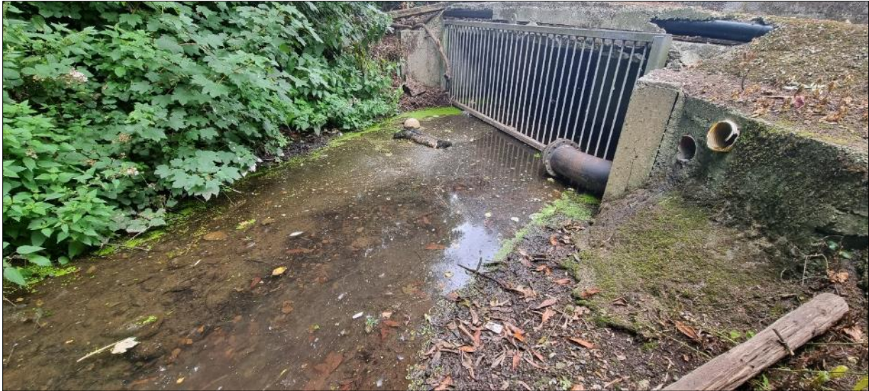
Plate 3.12 The Little Borris Stream at the culvert crossing of the Stradbally Road (N80) showing low summer flows and heavy siltation
