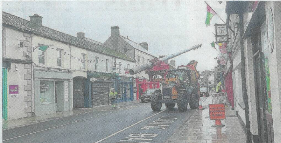
The old lighting poles were removed and replaced from Main Street last week. Picture: Pat Burbage
