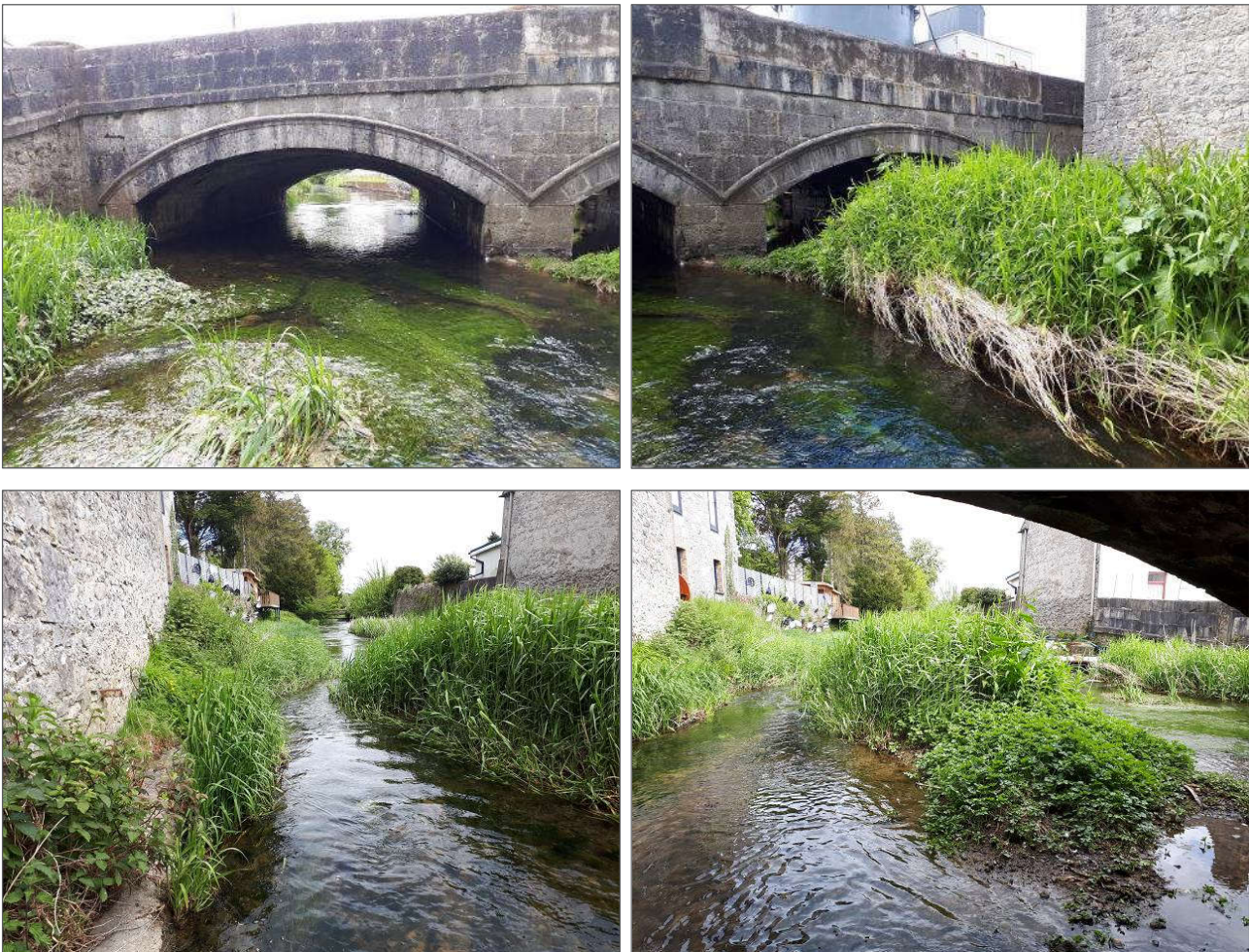
Plate 4.2 Immediately downstream of N80 bridge in Stradbally (May 2021).
