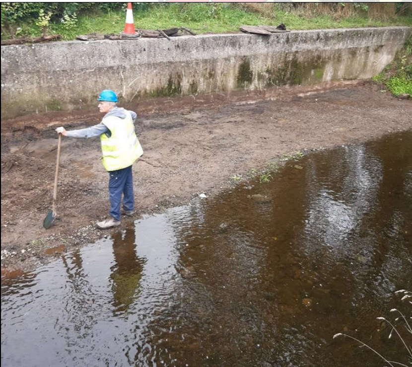
Figure 7 – Similar Area of silt reduced to water level.
