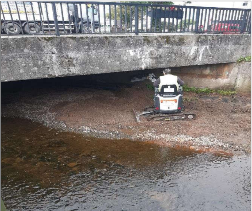
Plate 1.4 Example of similar works showing the small 1t excavator feeding silt material to suction line from the vacuum excavator truck (note the clean water adjoining the works).
