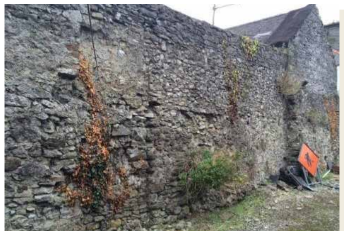
Fig.88: Detail of internal façade of west side of fort wall to the right of plate with later ope to left of plate
