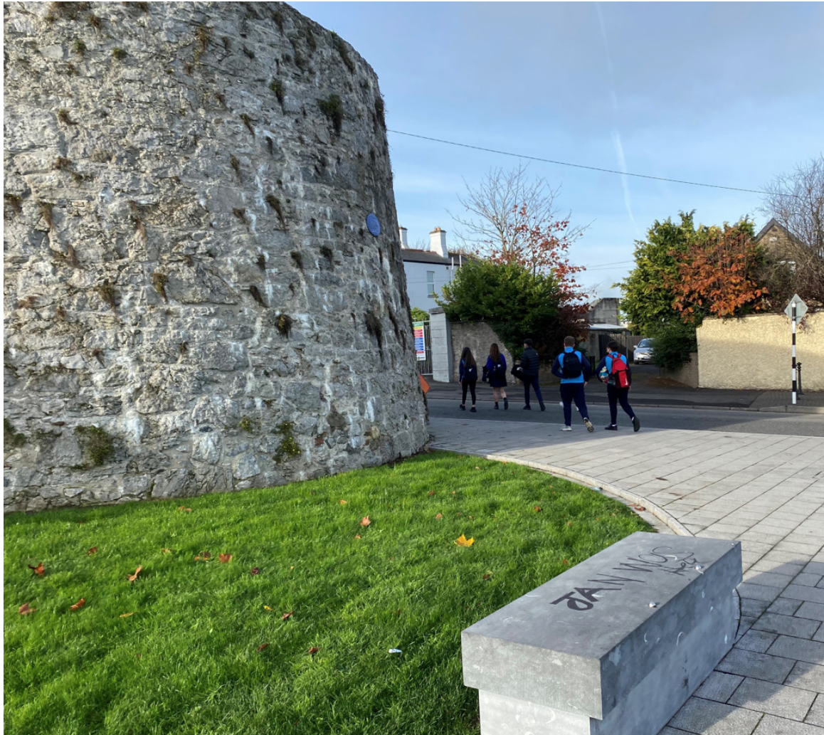
Fig.1.19: Photograph of the Circular Tower in its existing condition. Recent repointing visible.
