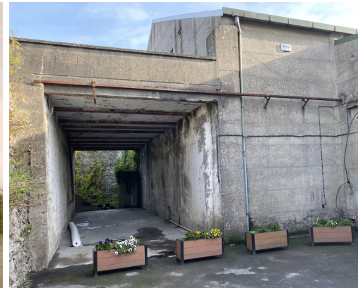
Fig.1.25: Concrete Structure to the north of the Granary Building, adjacent to the circular tower
