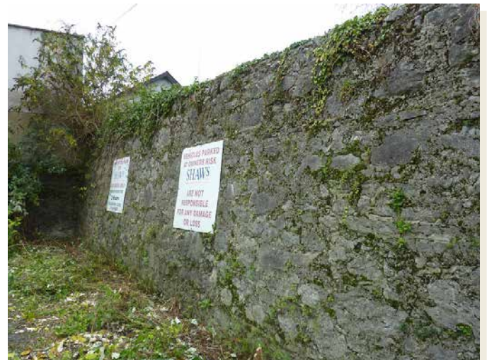
Fig. 101: View of external façade of fort wall in Site 18 from the east (Eoin Sullivan)
