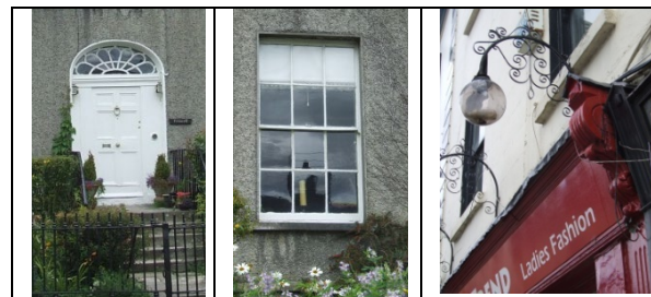
Surviving historic building fabric: painted timber door with decorative fanlight; timber sliding sash window with crown glass; decorative painted console
