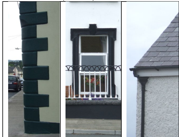
Building features: chamfered, faux quoins; raised plasterwork window surround with keystone detail and wrought iron railings to front; natural slate roof and cast iron hopper
