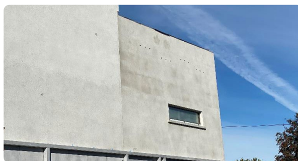
Swift bricks installed in the new library thanks to the work of BirdWatch Ireland (Laois branch) and Laois County Council
