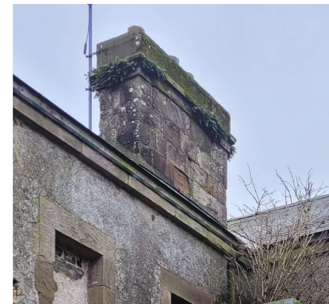
Chimney in poor condition
