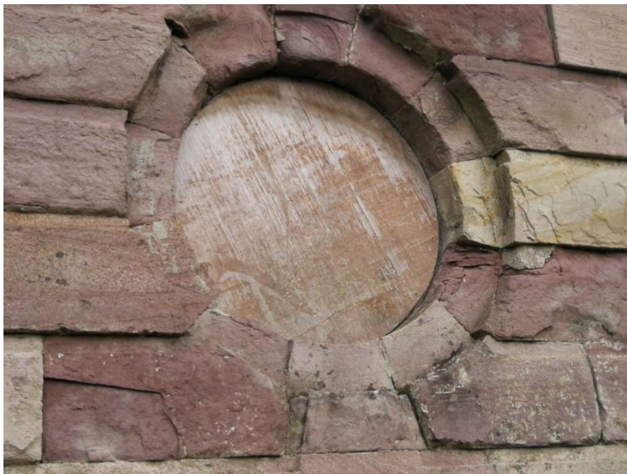
Figure 5 – Typical sandstone condition; spalling, cracked, falling away
