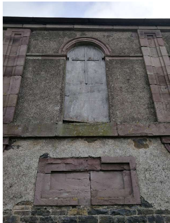
Figure 8 - Decaying sandstone, south elevation
