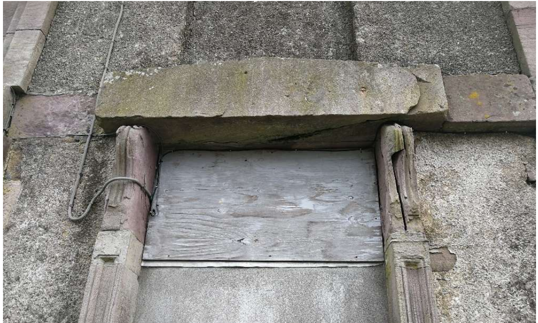
Figure 6 – Cracked lintel over door surround, west elevation
