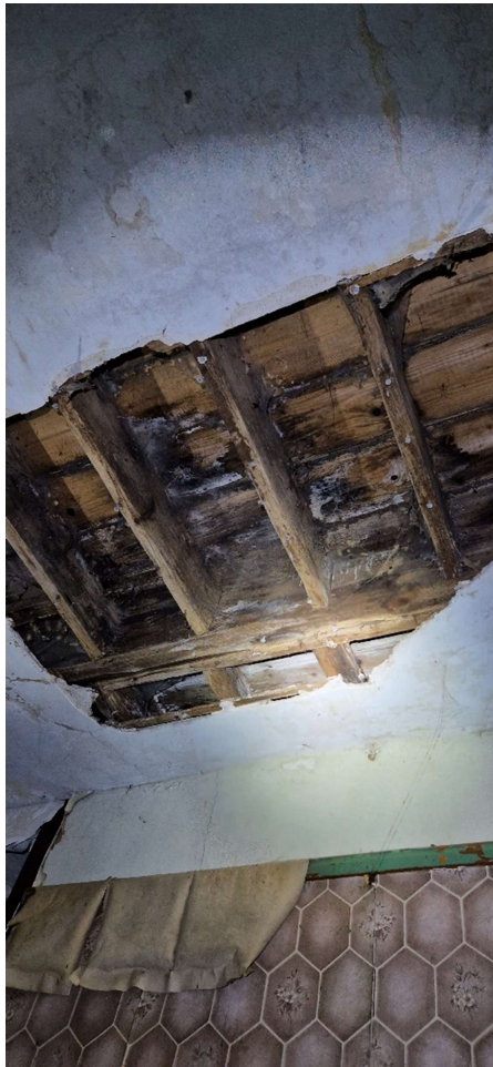
Figure 20 – Ceiling finishes missing in room GF-3
