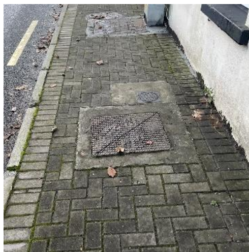
Poor quality surface finishes
