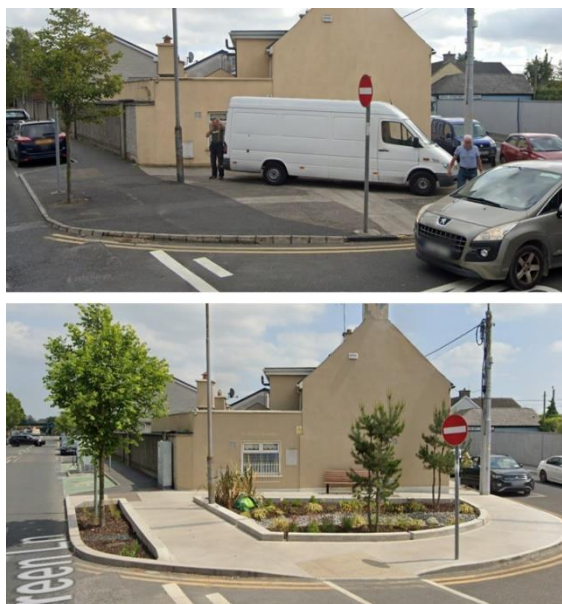
Figure 17-7 Before and After the installation of a Rain Garden at Green Lane / Pollerton Road, Carlow.
